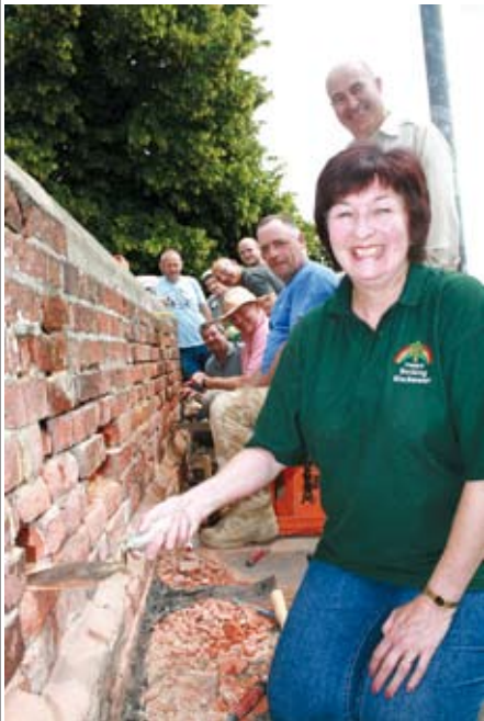
Wendy Schmitt with Mac Knox-Weir and course delegates get to work on the wall.
